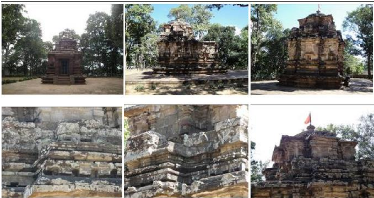
Figure 1 Front view, Lateral view and cross section of Mahadev temple, Bastar of Chhattisgarh showing fungal growth on the surface of Monument
